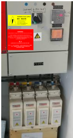
Main Switch for Electricity Account Meter
