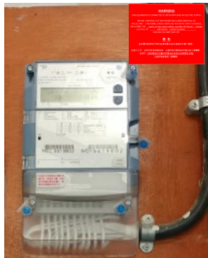
Electricity Account Meter
